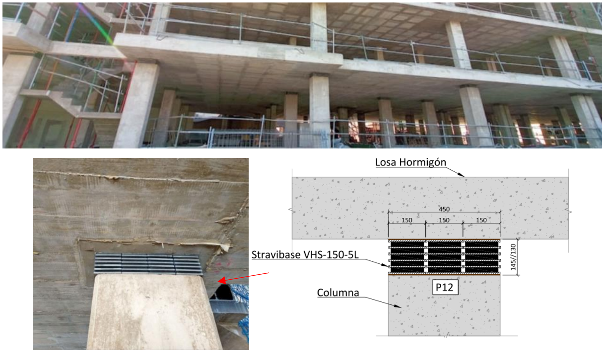
Figure 4 – Building decoupling using Stravibase VHS bearings.
