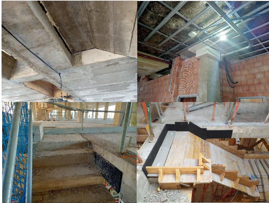
Figure 5 – Acoustic decoupling in the staircase, top of ground floor brick walls, and fire protection boards.
